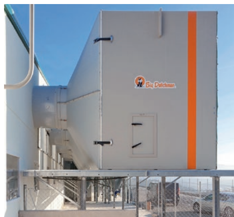
Installation for central fresh air distribution
